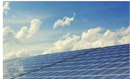
2. Mugharraq Port Warehouse 1,200 kWp
